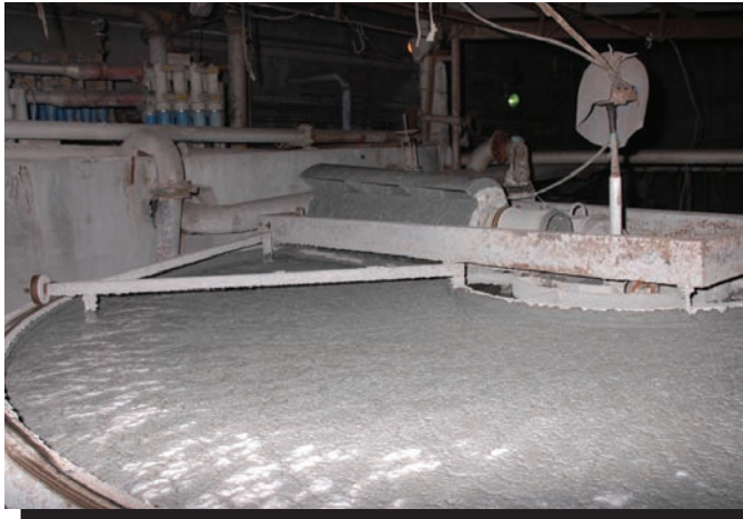
Effluent Treatment Plant
