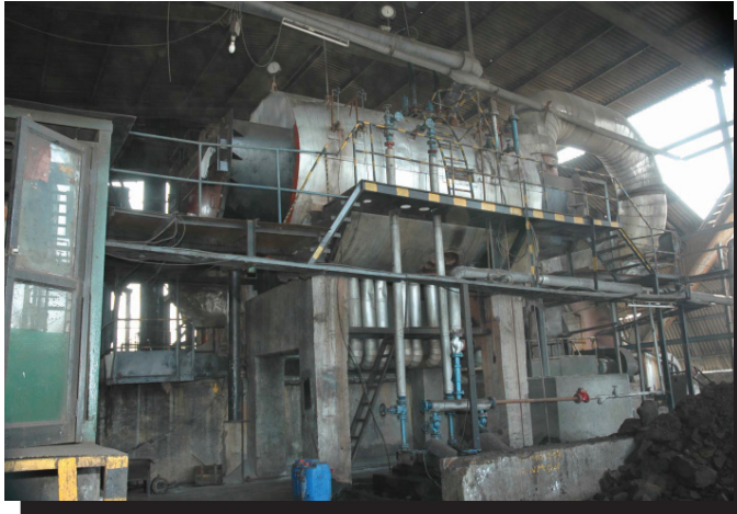
3MW Co-Generation Power Plant - Unit II
